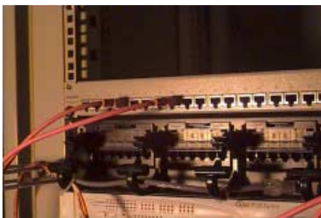
Figure 10: Hinged data closet frame containing switch and patch panel
